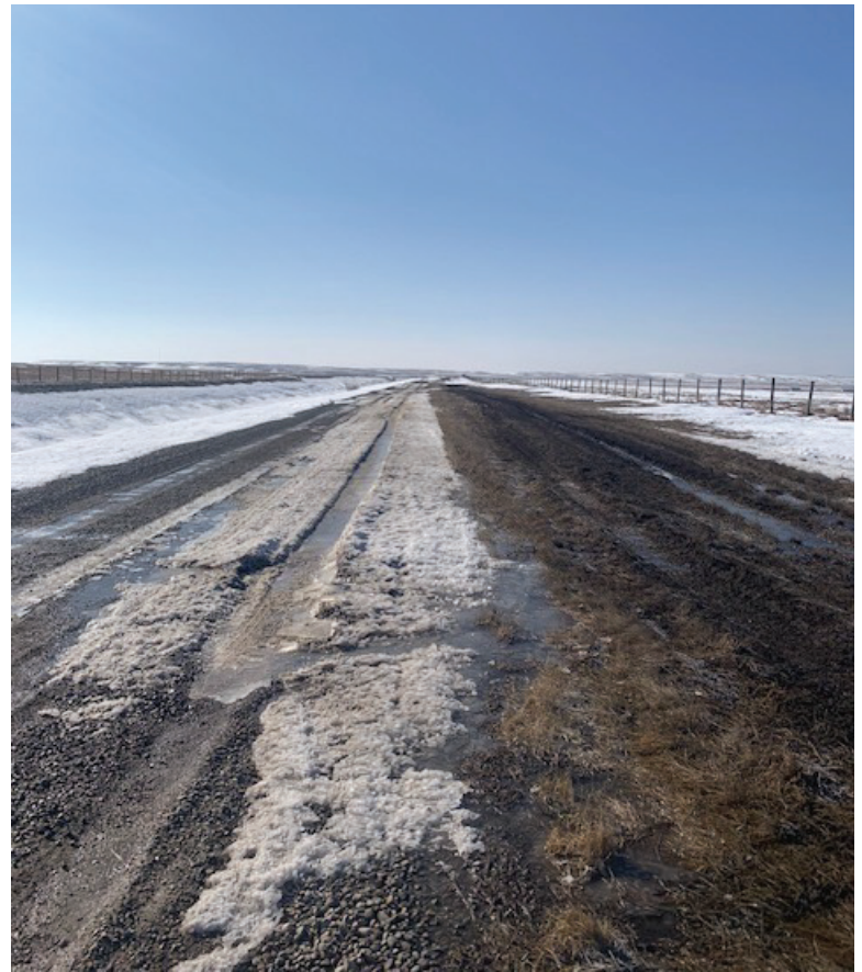
On the right side of the photo above, you can see damage caused by high traffic vehicles that use the canal service roads.
